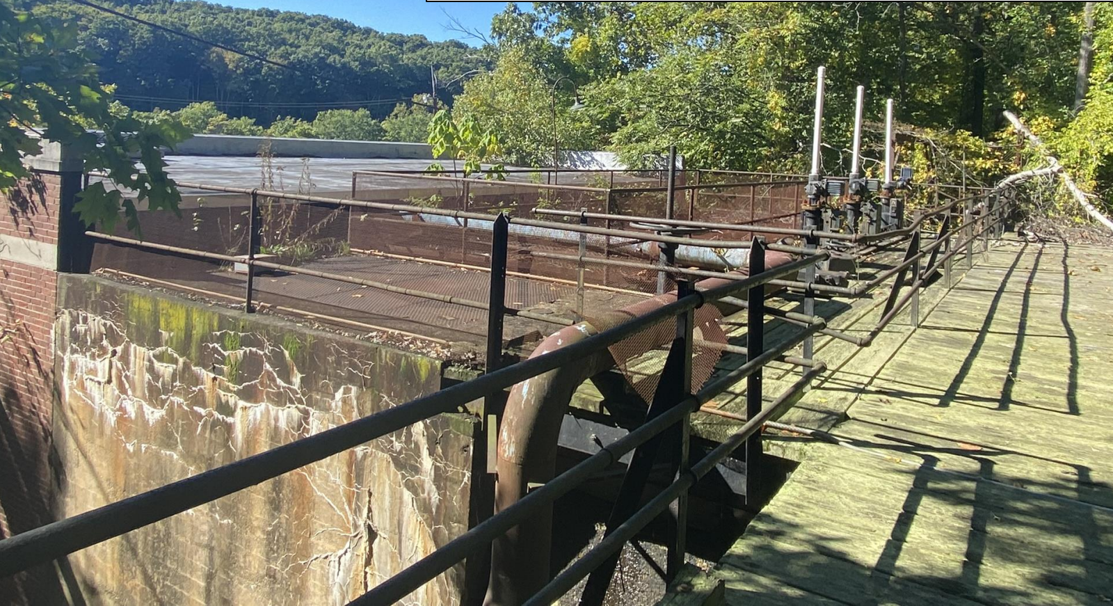
1 manual sluice gate and 3 mechanical sluice gates with screened intakes
