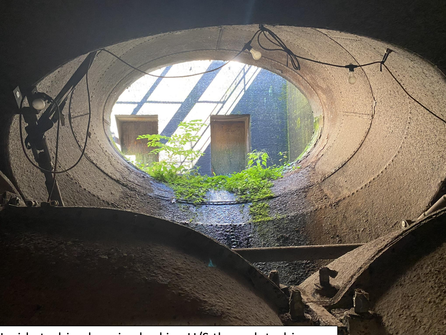
Inside turbine housing looking U/S through turbine intake pipe to forebay and outlets to 3 mechanical sluice gates
