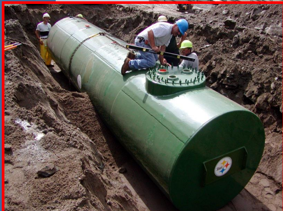
Underground Storage Tanks
