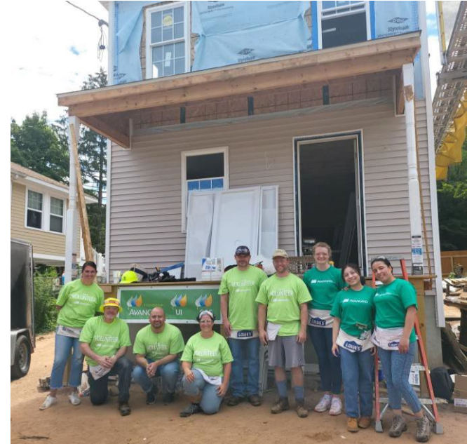
UI/AVANGRID employees volunteer at a New Haven Habitat for Humanity job site
