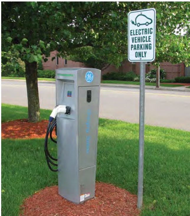
Electric Vehicle charging station, GE Plant, Plainville
