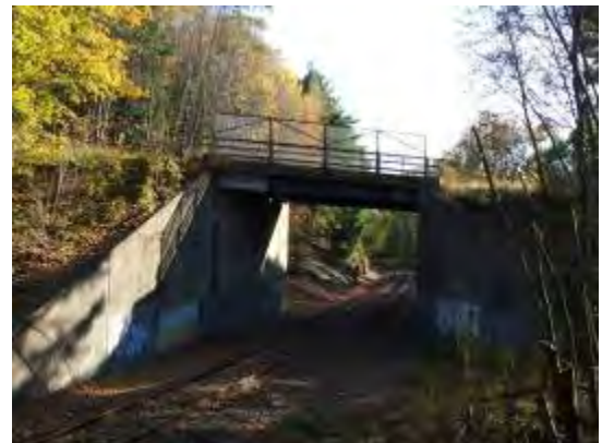
Existing Hill Road dry bridge over the railroad line just south of the Thomaston Dam.
